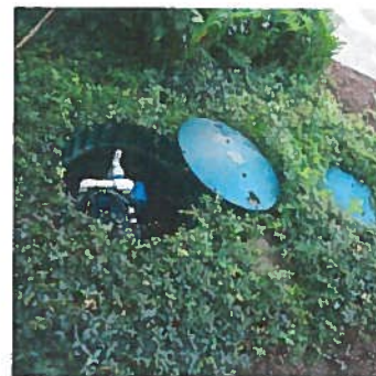
Figure 1: A resident of Lewes installed a 2,000-gallon cistern on site.
