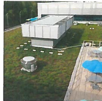
Figure 1: An example of a green roof installed on a commercial building is pictured above.
